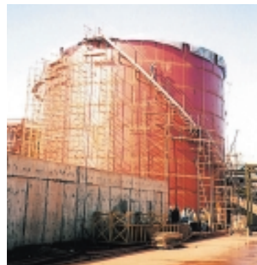
The anticorrosive rubber-lining project to the Coral Bay Nickel Corporation's nickel refining plant in the Philippines.
