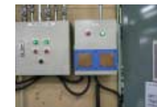
Measures to eliminate static electricity caused by human contact with the opening and closing of doors
