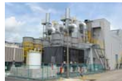
Cogeneration equipment at our Kuwana Plant
