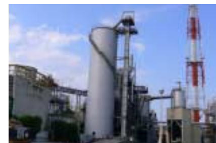
Cogeneration equipment at our Sendai Plant
