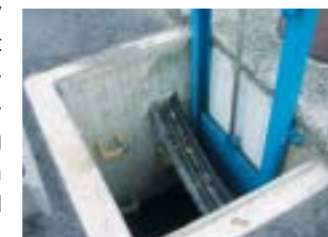
Emergency water interception valve at the final drain outlet of the plant
