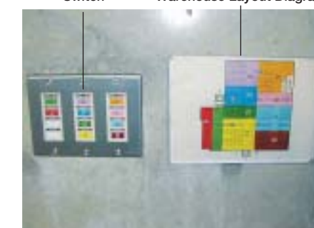
Positions of switches in the warehouse are broken down by colors to prevent turning on lights in unnecessary areas, thus promoting energy savings.
