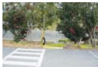
Water interception device installed at the drain outlet
