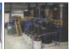
Wastewater treatment system
