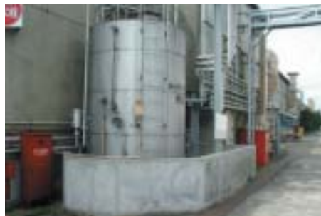
A dichloromethane storage tank with a protective wall
