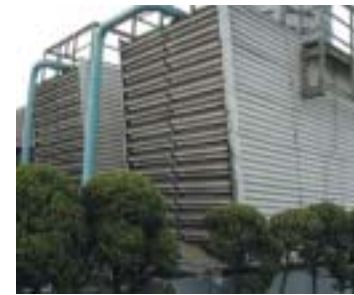
A water cooling and recycling facility
