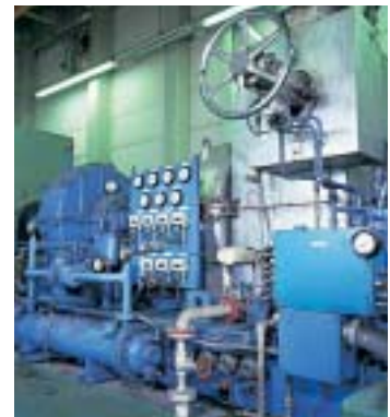
A cogeneration turbine at the Sendai Plant
