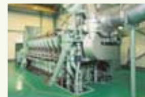
Cogeneration system operating at the Kuwana Plant
