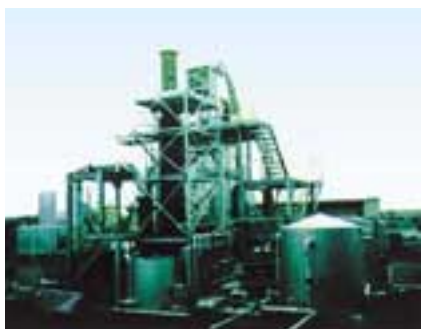
Stack gas treatment system installed on a mixed waste incinerator
