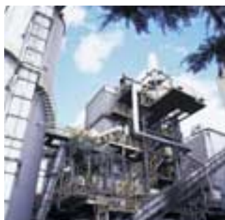
Cogeneration boiler equipped with a stack gas desulfurizer
