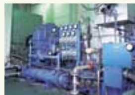
Turbine for the cogeneration system at the Sendai Plant
