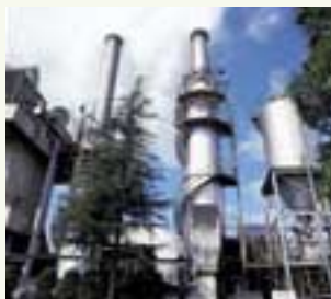
Cogeneration system operating at the Sendai Plant
