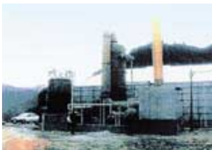
Deodorizing equipment eliminates odors in a poultry manure fermentation room
