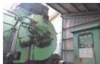
Energy-saving boiler (also serves as direct heating deodorizing equipment)
